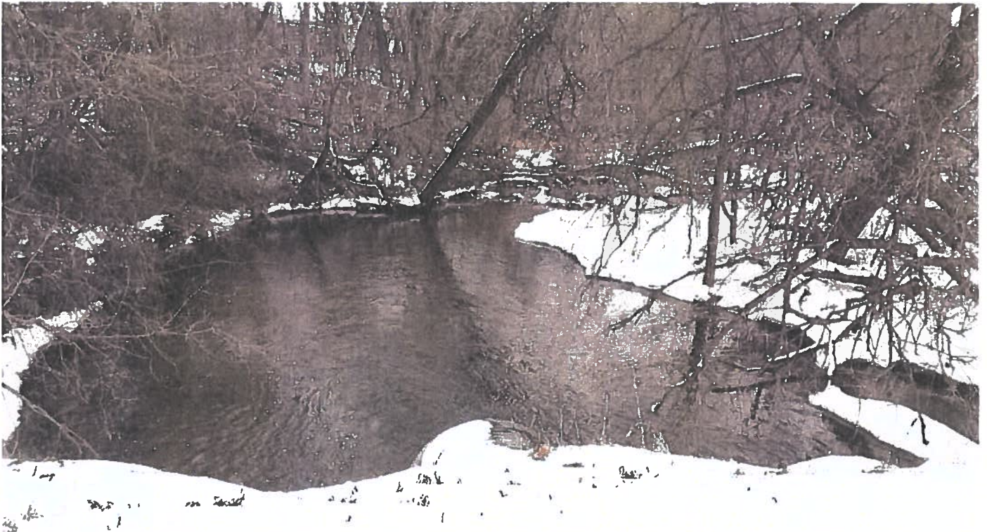
Existing CMP – Looking downstream (large scour hole)
